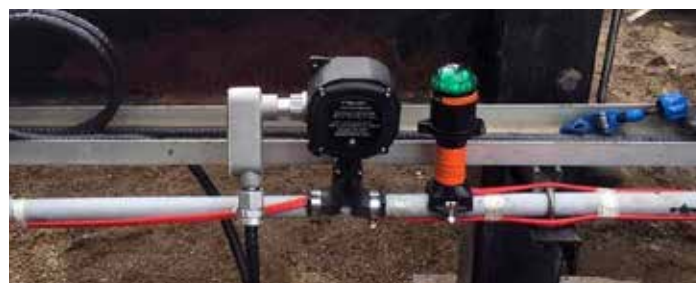
ProLine PTBO power connection kit and lighted end seal installed in industrial pipe trace application.
