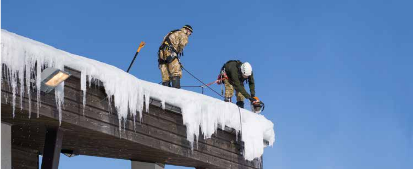
Shoveling and cutting down heavy, dangerous ice and icicles from the roof of a commercial facility.
