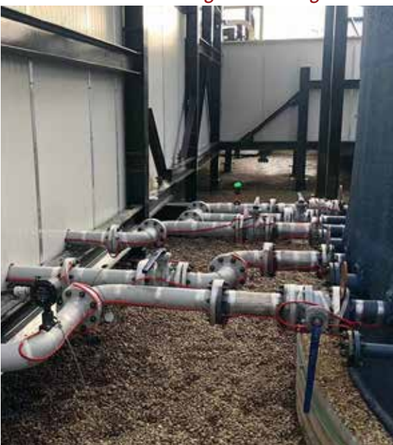
Pipe tracing system installed.
