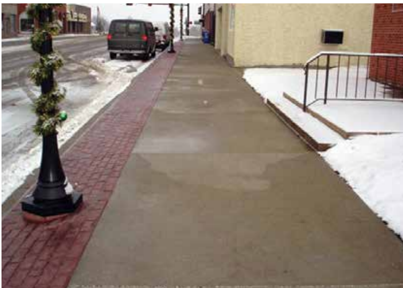
ProLine heat cable embedded in city sidewalks.
