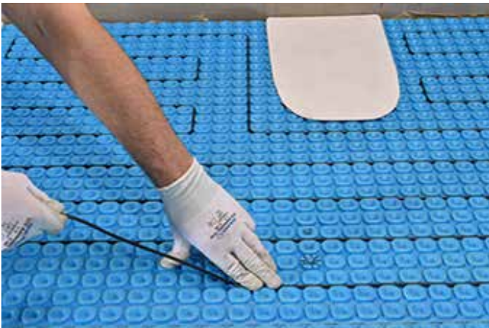
ProLine heat cable being installed in the channels of the Prodeso membrane.
