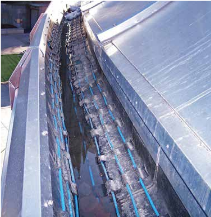
ProLine roof de-icing heat cable installed in commercial gutter heat trace application.
