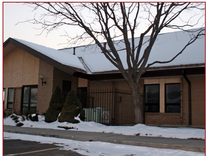
Commercial offices with the low-voltage roof heating system installed to heat the roof valleys and along the roof edges.
