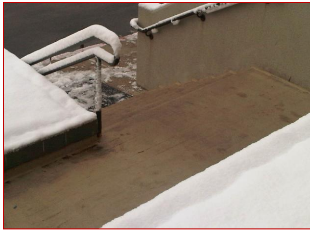
ProLine snowmelt system installed in concrete steps.
