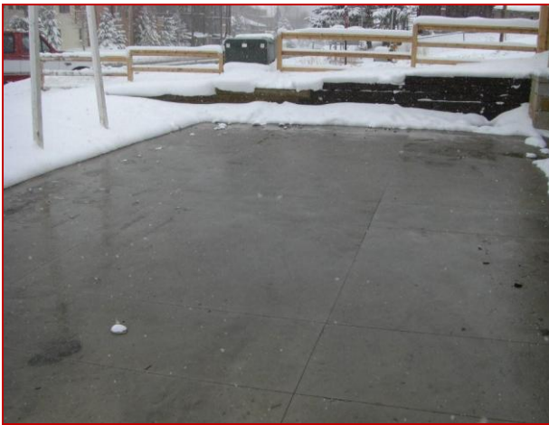
ProLine-heated concrete driveway and parking area.
