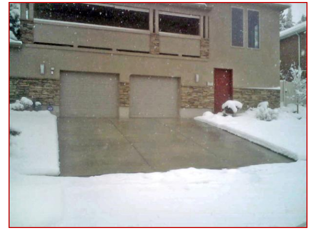
ProLine snow melting system in operation.
