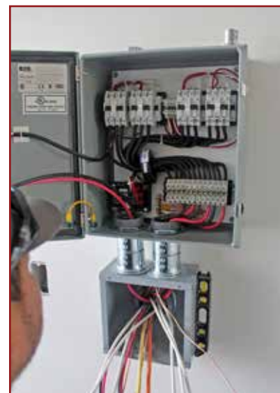
Contactor panel being installed.
