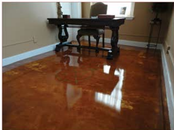
Floor heating system installed in stained concrete.
