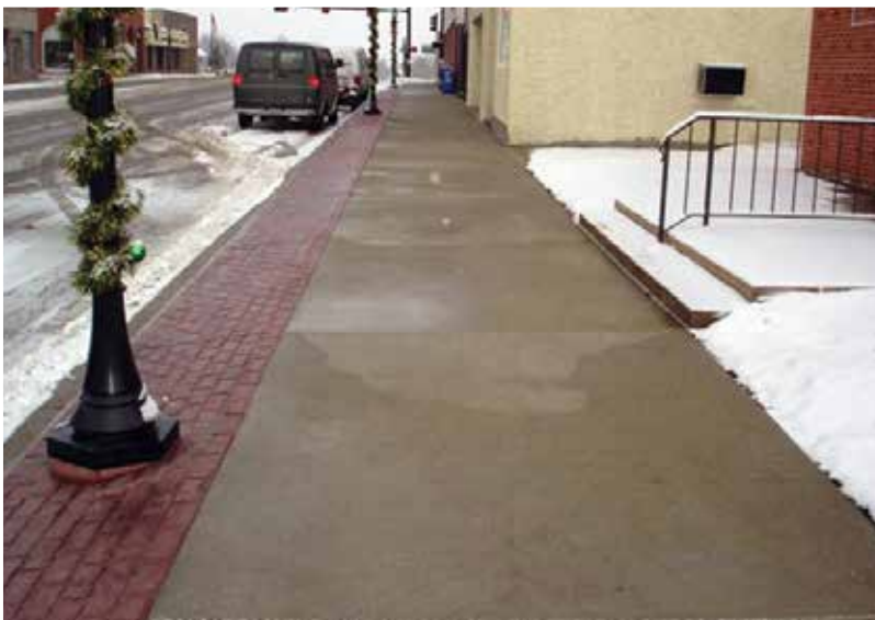
Snow melting system installed in city sidewalks.
