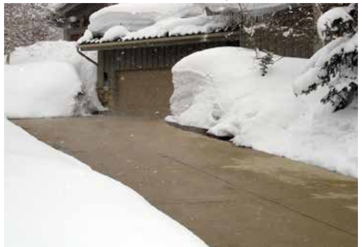
Radiant heated driveway.
