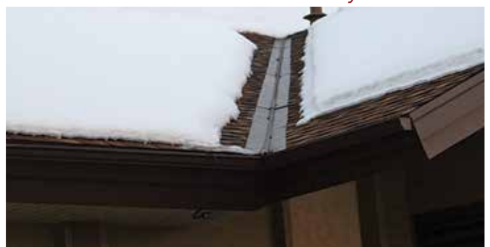
Low-voltage roof deicing system heating roof valley and edge.
