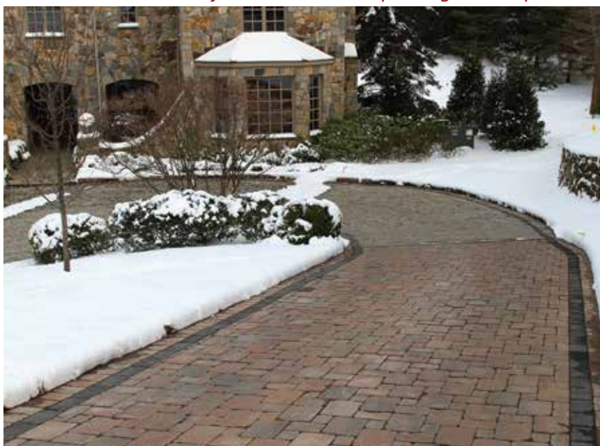
Snow melting system installed in paver driveway.
