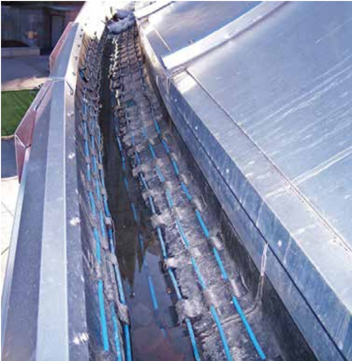
Roof deicing heat cable installed in commercial gutter heat trace application.
