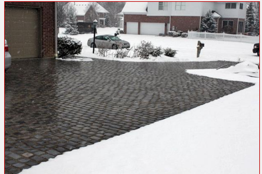
AFTER: ProLine snow melting system in operation.
