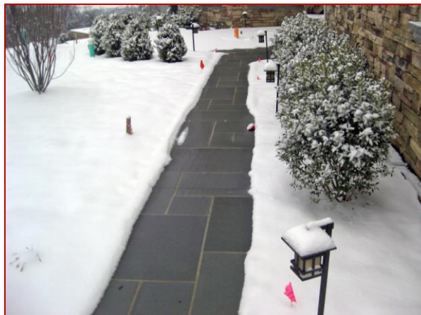
ProLine snow melting system installed under paver sidewalk.
