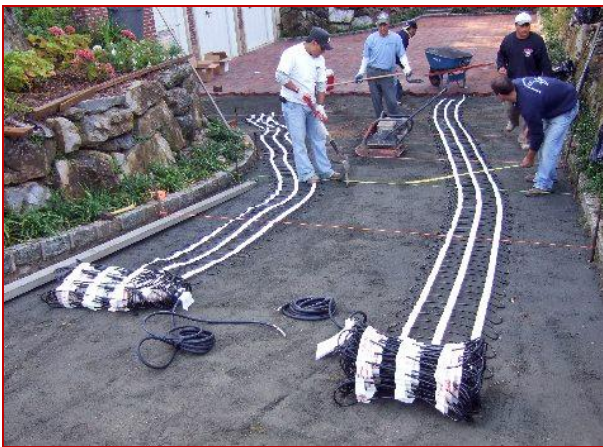
ProLine snow melting mats being installed for heated paver tire track driveway.
